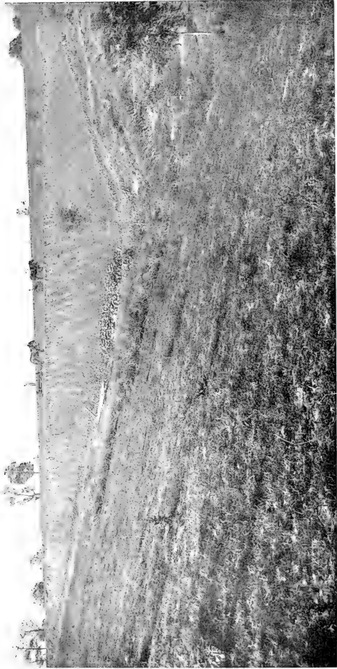
Courtesy U. S. Geological Survey. CONSTRUCTING AN EARTHEN RESERVOIR EMBANKMENT, COLUMBIA, MO.
